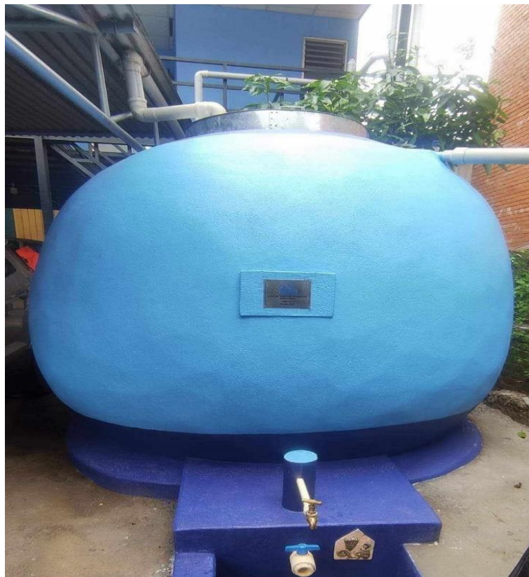
Fig. 1: Photo of pumpkin-shaped RWH Tank
